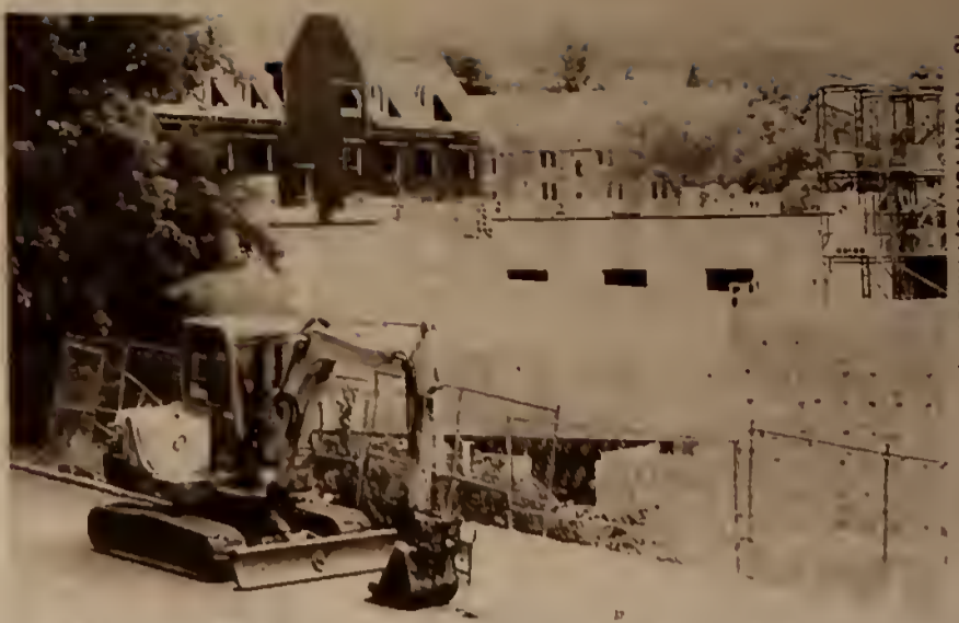
IVY AWAITS THESE WALLS: The foundation and basic shape of Whitman College on the former tennis courts on the Princeton University campus are starting to take form. The school was named for eBay CEO Meg Whitman, the principal sponsor in the project, after she donated $30 million to the University in 2002.
