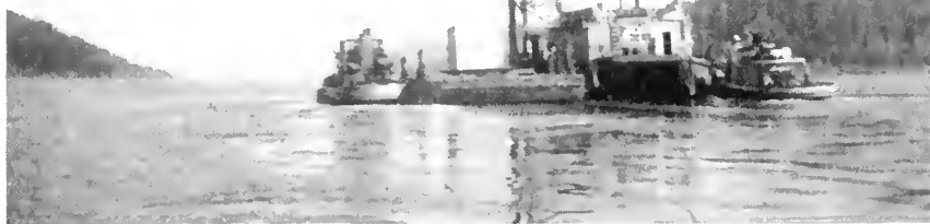
Huge drilling scow, a little city in itself, shown with tugs in moment of quiet water in one of the world's swiftest tide races. A new anchor is being dropped, weighing 75 tons. Six anchors, totaling 550 tons, held it only temporarily as 11 steel cables kept breaking through "fatigue" caused by movement of scow in shifting water.
