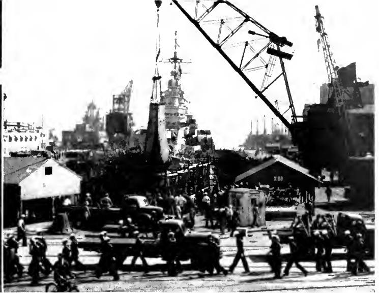
Final keel section goes into place on the Pittsburgh. Communications, piping and wiring are already installed in the previously-fitted portions. (Official U. S. Navy Photograph).
