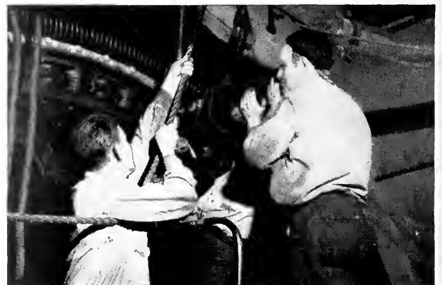
Removing field coil from the rotor for cleaning and inspection. Skilled G-E workmen with years of specialized marine experience stand ready to help you get fast, reliable ship-board repairs and save days of unprofitable port time.
