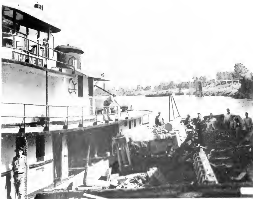
The new Cooper-Bessemer JS-8 supercharged diesel slips into the engine room by means of chain hoists, wire rope, some manpower and plenty of ingenuity on the part of Houglan's port engineer, W. B. Hassell.
