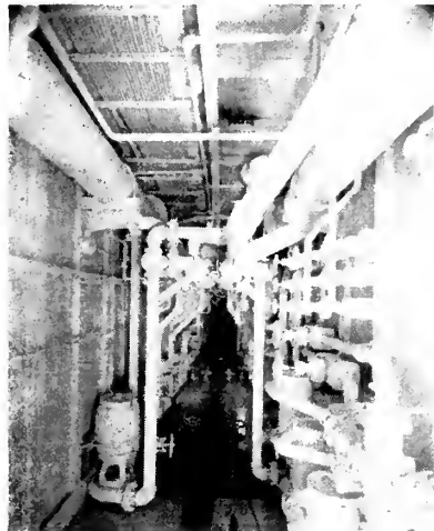
Brine pumps and piping in passage between bait and fish holds.
