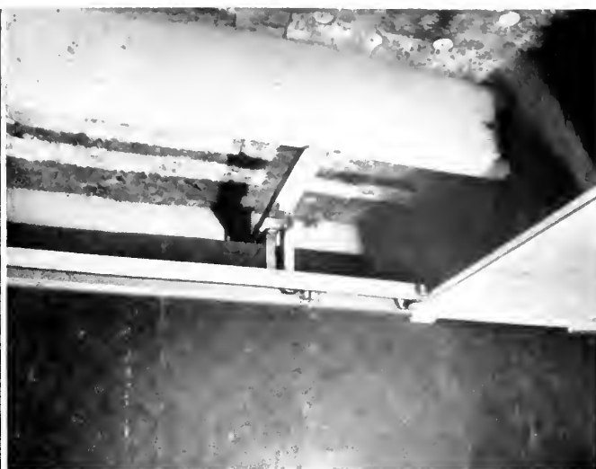
Fig. 2. Close-up of Aetna ceiling structural shapes in place securing flush bulkhead panels and marinite ceiling panels.
