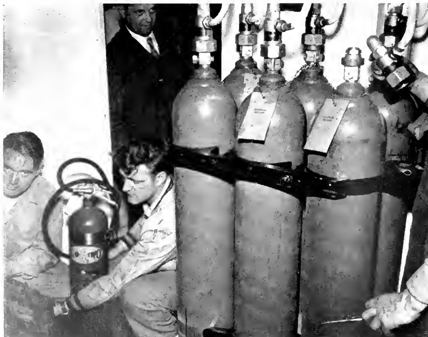
PMR's camera caught this Ets-Hokin Galvin crew in action, installing C-O-Two Fire Equipment unit on the tuna vessel White Star at San Francisco during March. The White Star will be featured in the May Pacific Marine Review.
