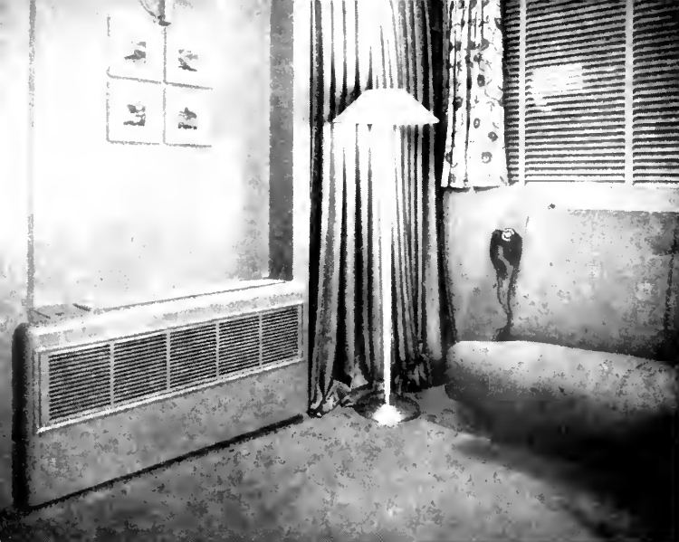
Fig. 5. View of high pressure primary air induction unit, in large cabin class stateroom. (Courtesy Aetna Marine Corp.)
