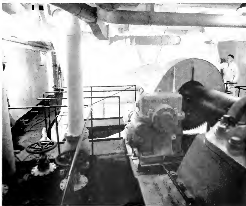
One of the 10,000-hp propulsion motors. Completely enclosed, these synchronous motors are cooled by a recirculating air system and the heat is released to the atmosphere through a surface air cooler.
