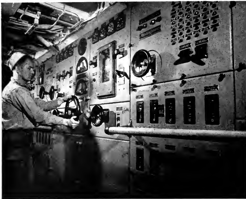
Propulsion control and auxiliary switchboard.
