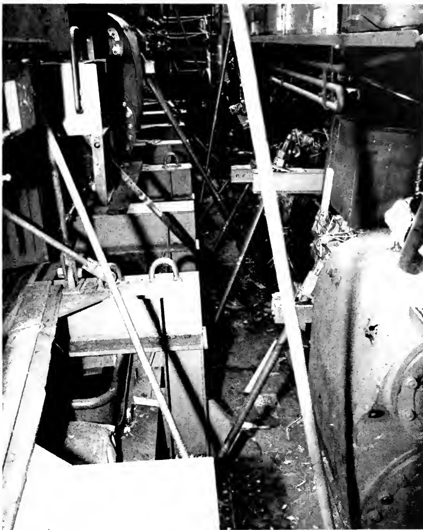
Supports over hatch and hold down fastenings.
