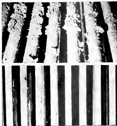
Upper view shows typical hard combustion deposit on boiler tube section. Lower view illustrates boiler tube section after application of gamlenite.
