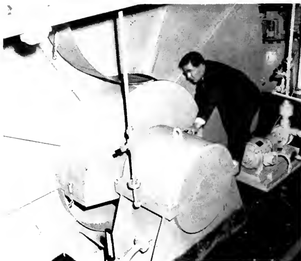
John Baer, port engineer at Los Angeles, is shown inspecting brushes on a 3300-hp main motor aboard an APA-type Navy transport.
