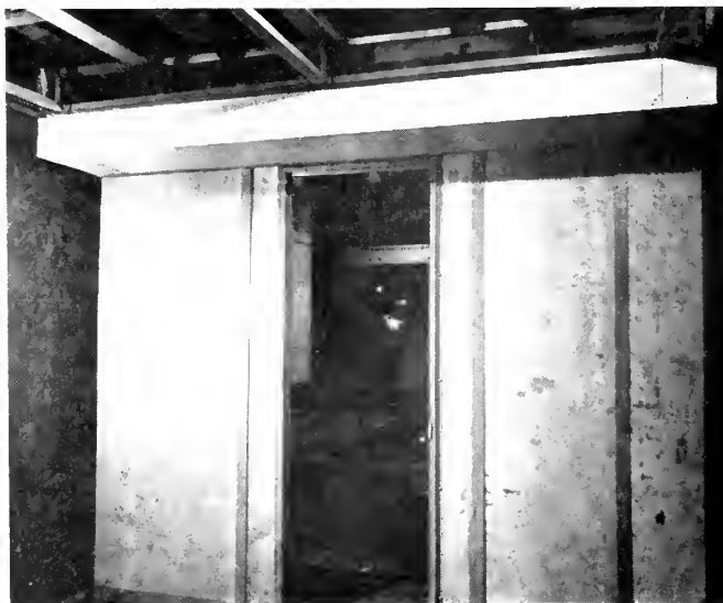
Fig. 3. Aetna joiner door frames installed ready for hanging of door. Ceiling structural members installed with offset, to meet special condition, ceiling panels in place on offset.
