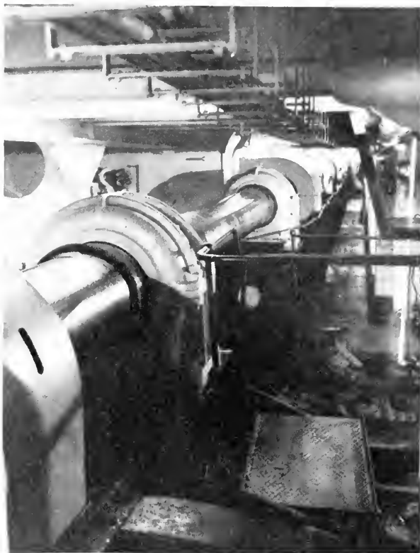
Shaft alley of the USS LeJeune, showing one of her propeller shafts. After 18 Atlantic crossings these bearings showed no measurable wear. Each is 15 \frac{3}{8} inches diameter, delivers 750 hp, and is mounted on 13 bearings.
