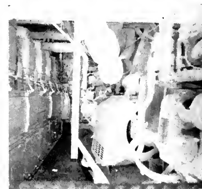
Main Enterprise Diesel engine and Caterpillar Diesel-driven generator and pump.
