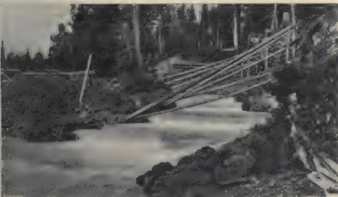
The Fish-way at Meziaden Falls, Naas River watershed, B.C. The cross timbers shown brace the retaining wall to prevent ground from filling the basins.
