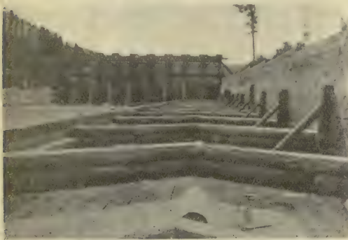
Looking up the race at Quesnel Dam, showing the construction of the fish-way on the floor of the race. The gates being closed.
