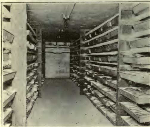
3.—The New Brunswick Cold Storage Co., Limited, St. John, N.B. One of the five sharp freezers, with pans.
